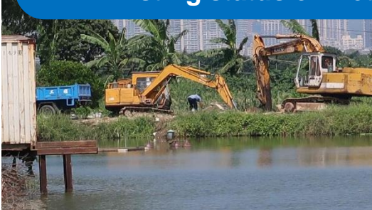
Unauthorized pond filling
